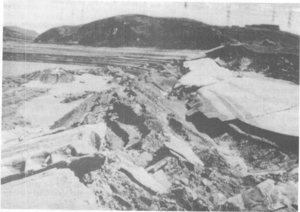
Figure 3. Slumping of the Lower San Fernando Dam in the 1971 San Fernando earthquake.
