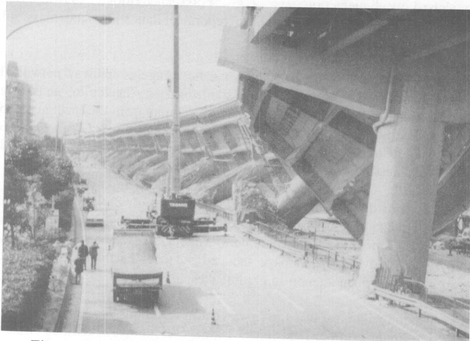
Figure 5. Collapse of Hanshin expressway during the 1995 Kobe (Hyogo-Ken Nabu, Japan) earthquake.
