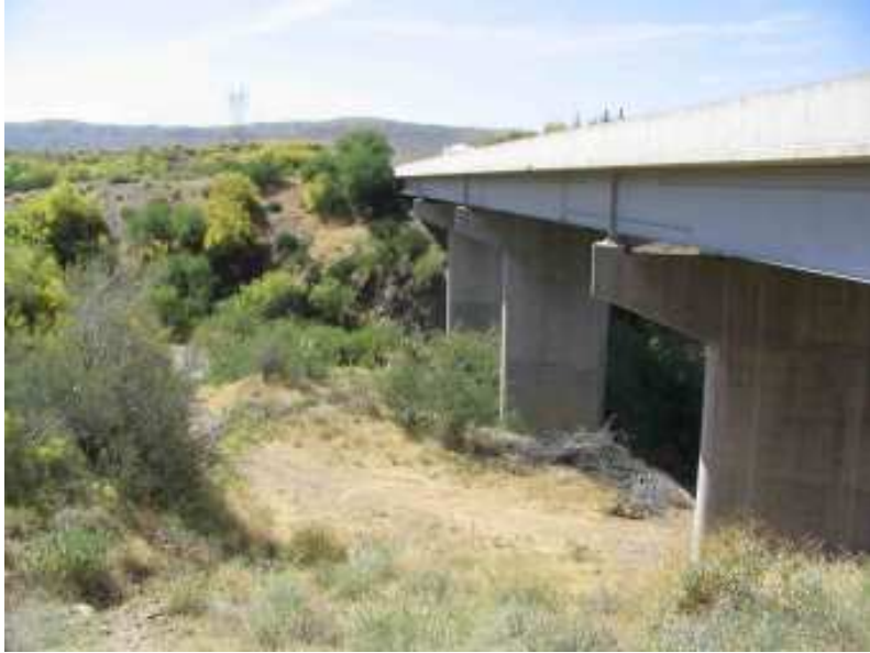
Figure 5. Little Squaw Creek Bridge, constructed in the 1960's, is a 2-lane, 5-span, 315-foot (96 m) long bridge constructed of reinforced concrete. The structure is supported on spread footings at both the south abutment and pier locations. Seismic lines were completed at or between Piers 1 and 2 in or near the active channel. Equipment was hiked into the small canyon from the vehicle parked by the highway.
