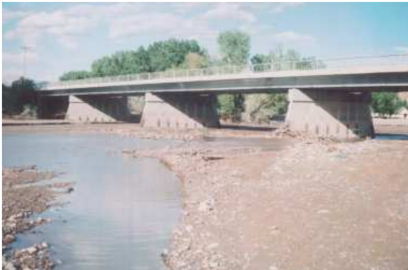
Figure 1. Beaver Dam Wash Bridge (Piers 2, 3 and 4) in Northwest Mohave County, Arizona after winter 2005 flood. Surface seismic lines were completed between each set of piers and abutments. Surface resistivity was completed at a previously installed piezometer on a gravel bar in the northern portion of the stream channel bed.
