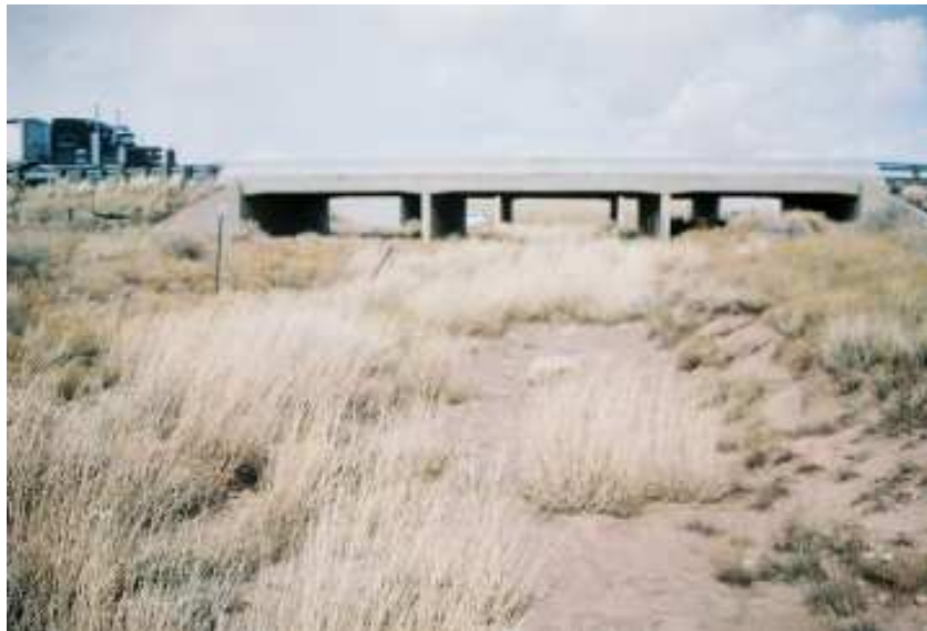
Figure 8. East-bound Babbitt Tanks Wash Bridge is in foreground looking north. Piers 1 and 2 are located in or adjacent to the active channel of Babbitt Tanks Wash. Based on the 1944 plans, pier foundations are three-foot (0.9 m) wide strip footings that are 18 inches (0.46 m) thick. Plans showed footing bottoms set approximately six inches (0.15 m) below the "Probable Solid Rock Line."
