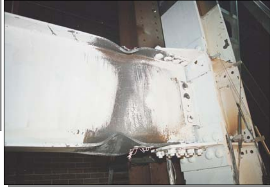
Plastic hinge formation -- flange and web local buckling
