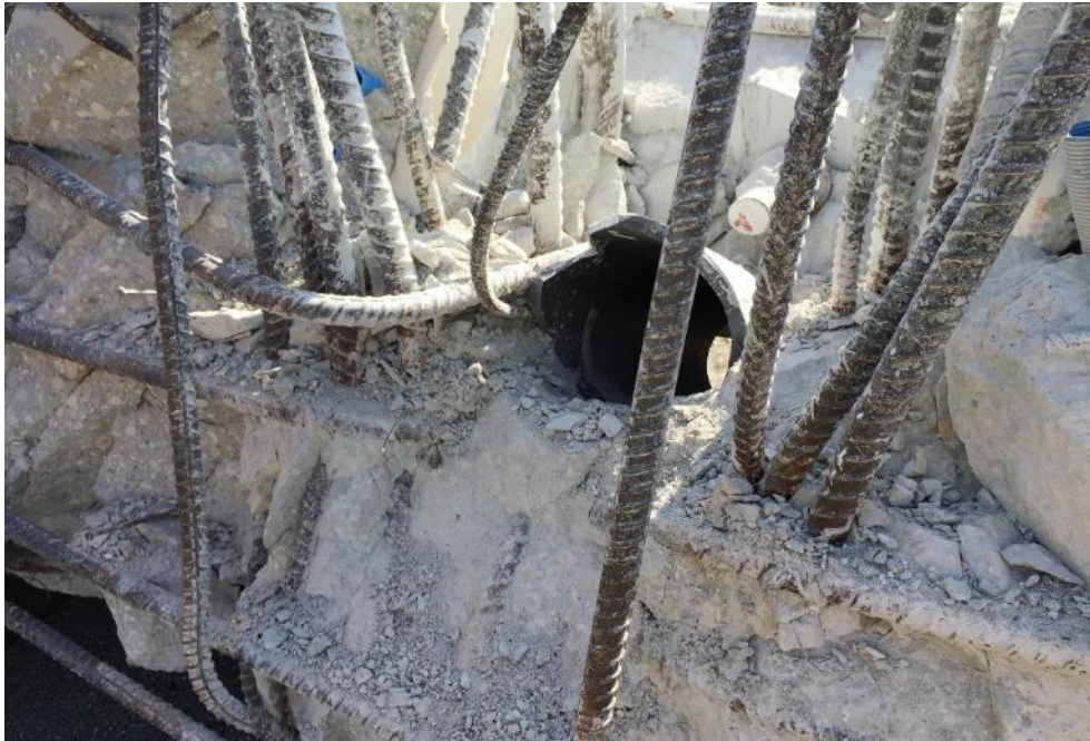
Figure 68 Punched hole in Diaphragm II at the time of the bridge collapse – from south looking towards north, April 9, 2018, by OSHA
