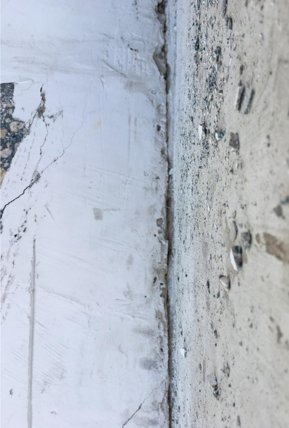
Figure 37 Cracks at the construction joint of the main span deck and diagonal 11 on 3/13/2018 by BPA
