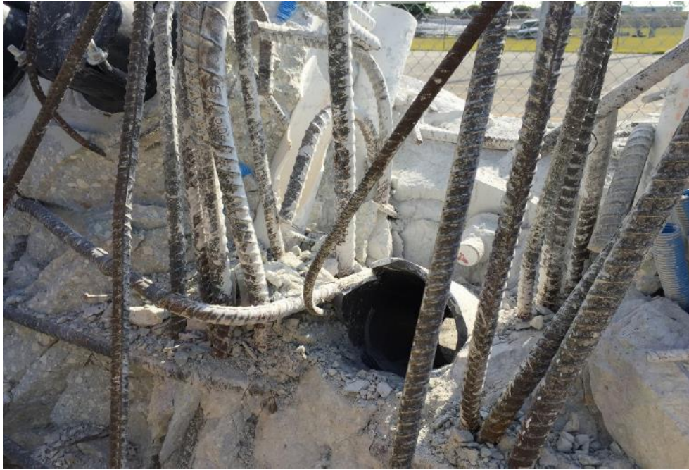
Figure 70 Punched hole in Diaphragm II at the time of the bridge collapse – from south looking towards north, April 9, 2018, by OSHA
