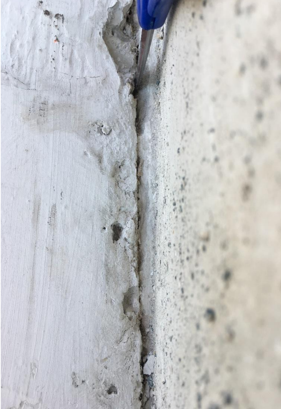
Figure 33 Cracks at the construction joint of the main span deck and diagonal 11 on 3/13/2018 by BPA
