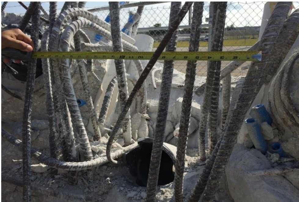
Figure 69 Punched hole in Diaphragm II at the time of the bridge collapse – from south looking towards north, April 9, 2018, by OSHA
