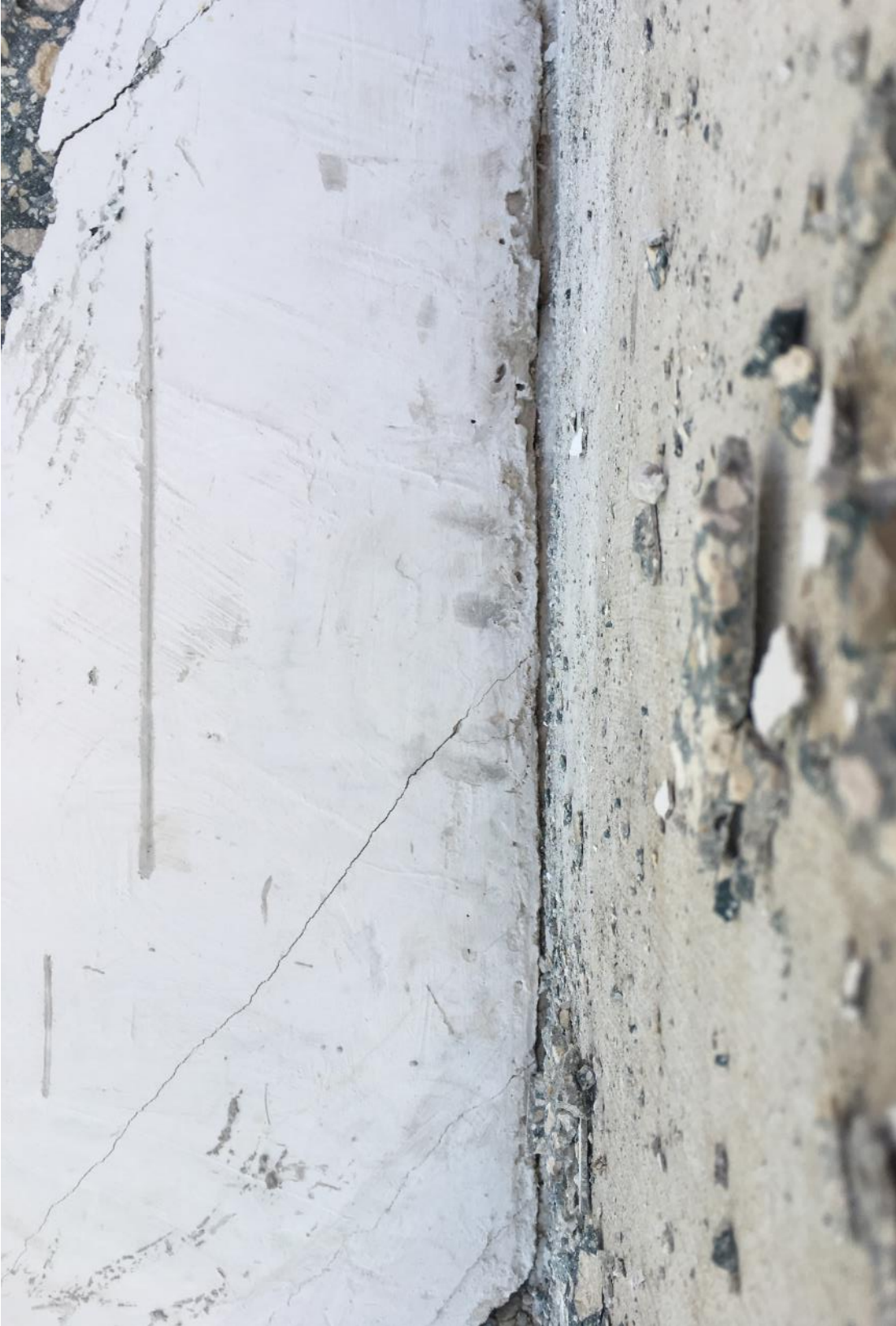
Figure 36 Cracks at the construction joint of the main span deck and diagonal 11 on 3/13/2018 by BPA
