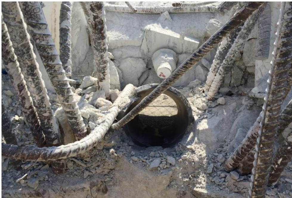
Figure 67 Punched hole in Diaphragm II at the time of the bridge collapse – from south looking towards north, April 9, 2018, by OSHA
