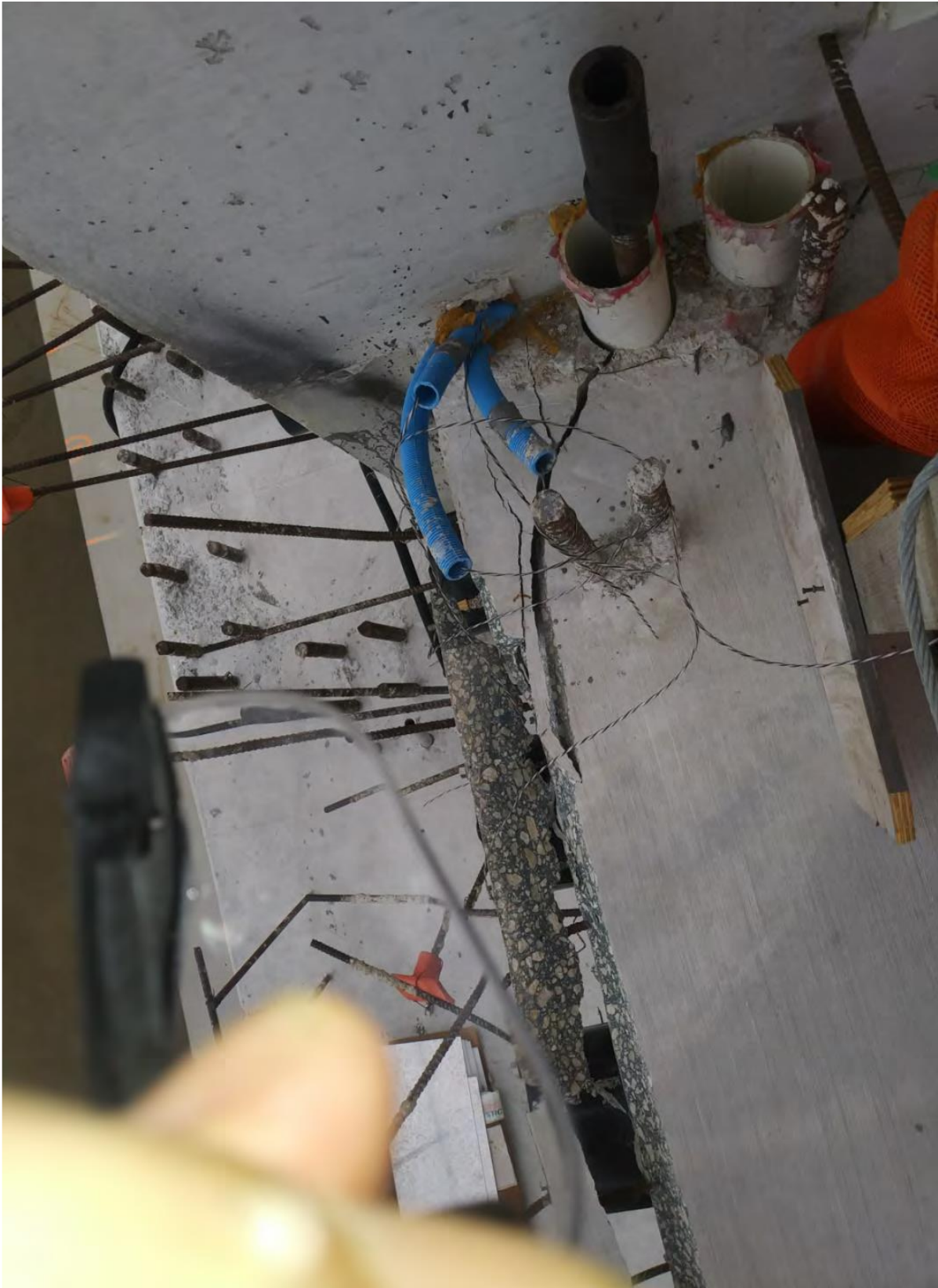
Figure 24 Cracks at the west side diaphragm II MCM email of 3/12/2018 – top face, by BPA.
