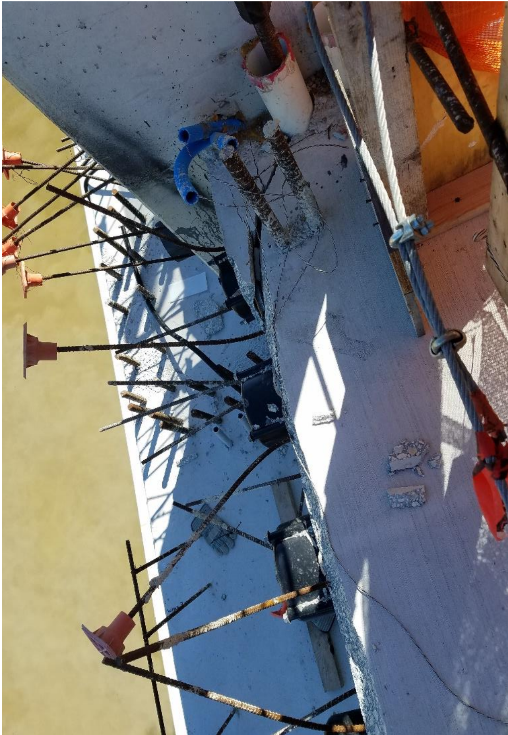
Figure 28 Diagonal cracks on the west side of diaphragm II on 3/13/2018, by BPA – top face
