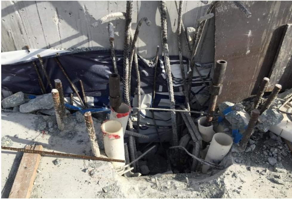
Figure 58 Concrete blow-out failure in Diaphragm II at the time of bridge collapse at the site looking north from south, March 21, 2018, by OSHA
