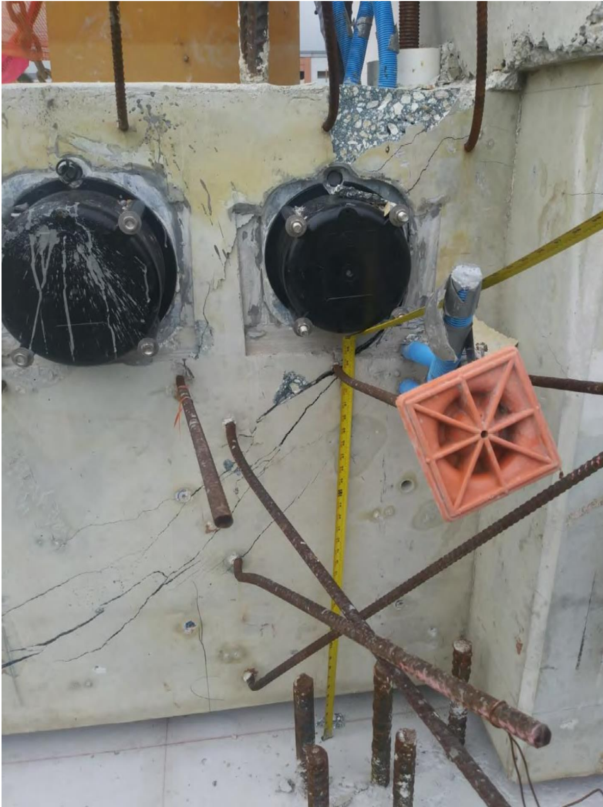
Figure 27 Cracks on the east side diaphragm II MCM email of 3/12/2018, by BPA – side face
