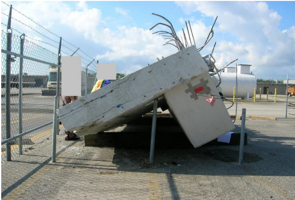
Figure 71 Side view of the saved portion of the diaphragm II in storage yard, April 9, 2018, by OSHA
