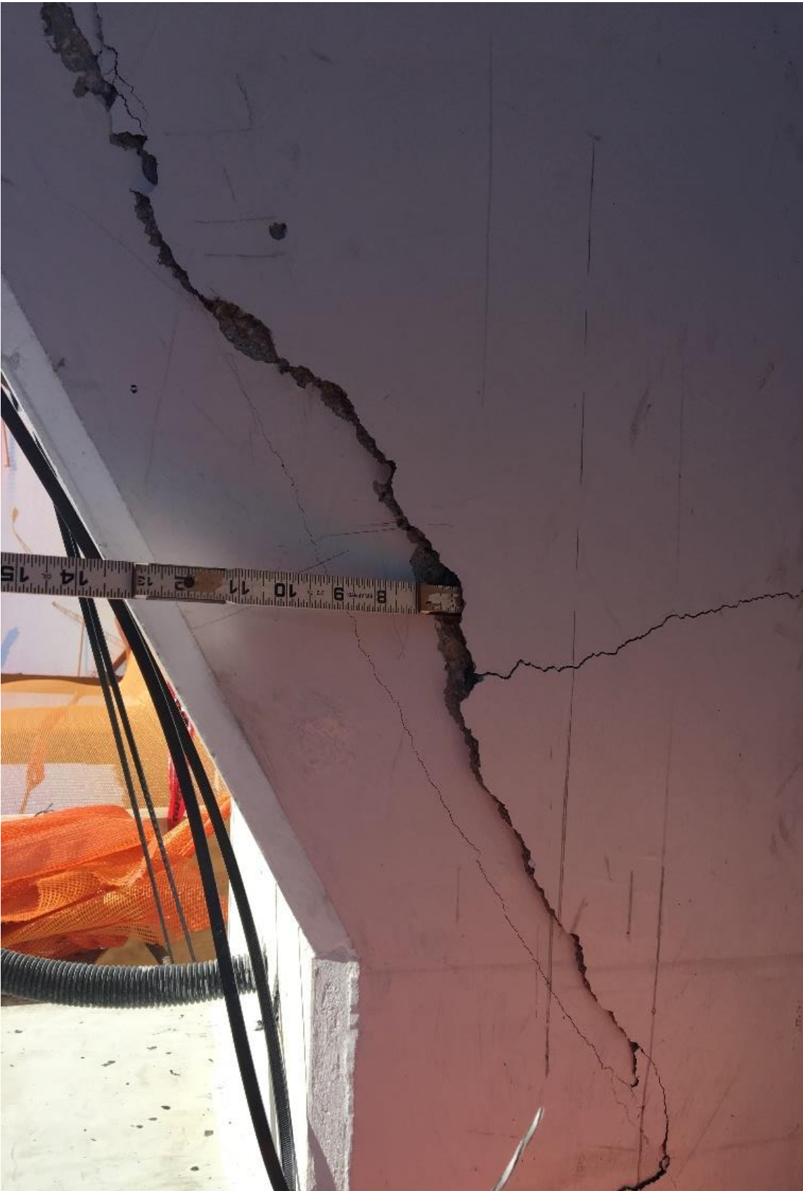
Figure 39 Close-up of longitudinal cracks in diagonal 11 on 3/14/2018 by BPA
