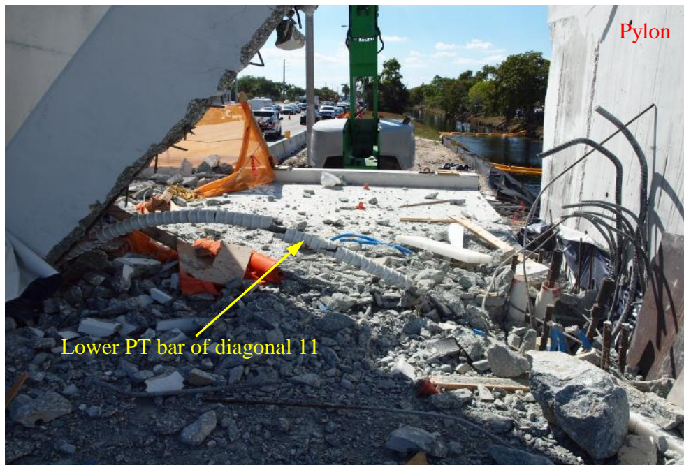
Figure 57 Lower PT separated from the diagonal 11 still embedded in diaphragm after bridge collapse, March 17, 2018 by OSHA
