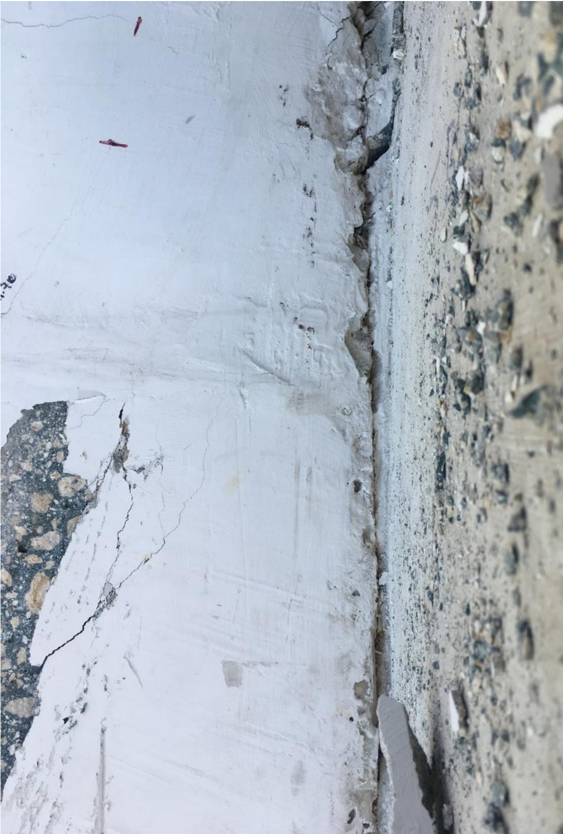
Figure 38 Cracks at the construction joint of the main span deck and diagonal 11 on 3/13/2018 by BPA
