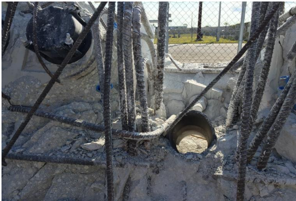
Figure 65 Punched hole in Diaphragm II at the time of the bridge collapse – from south looking towards north, April 9, 2018, by OSHA
