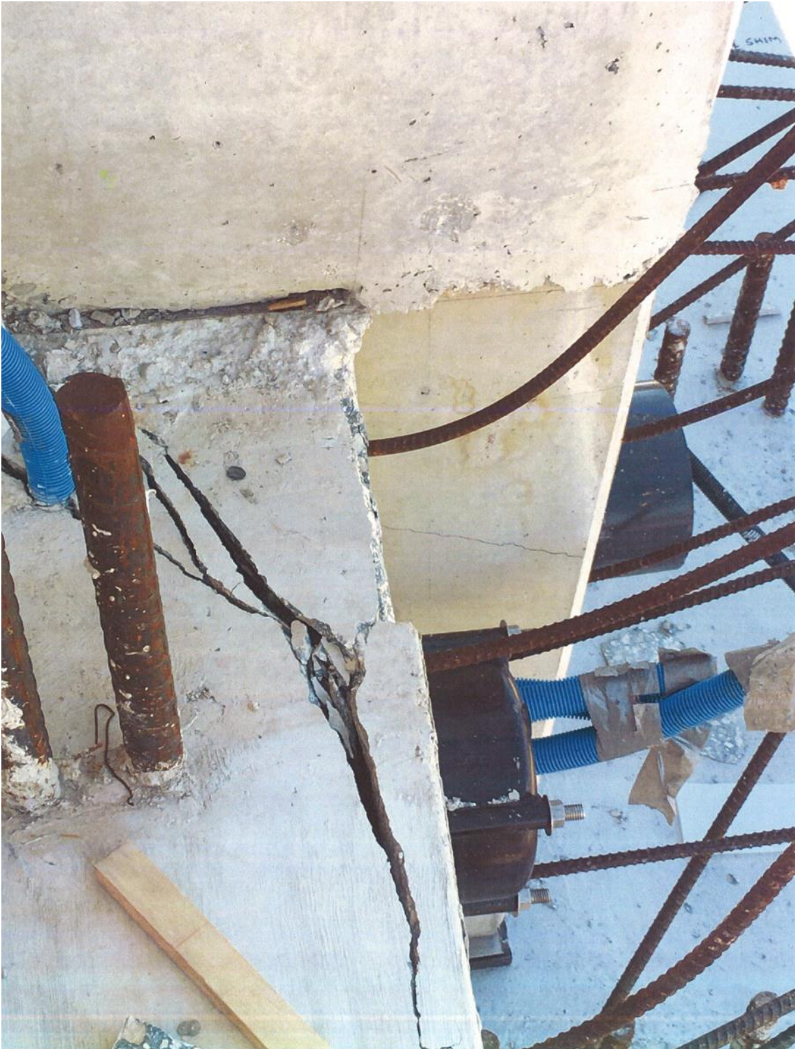
Figure 44 Cracks and movement of the column at the east side of diaphragm II on 3/14/2018 by BPA
