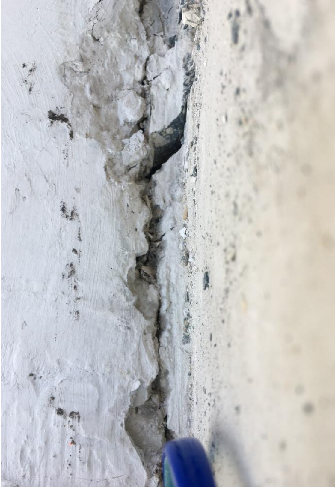
Figure 32 Cracks at the construction joint of the main span deck and diagonal 11 on 3/13/2018 by BPA
