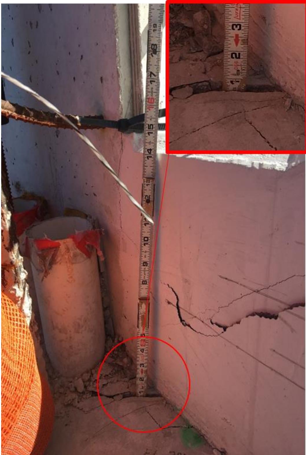
Figure 42 Cracks at the west side of diaphragm II on 3/14/2018 by BPA
