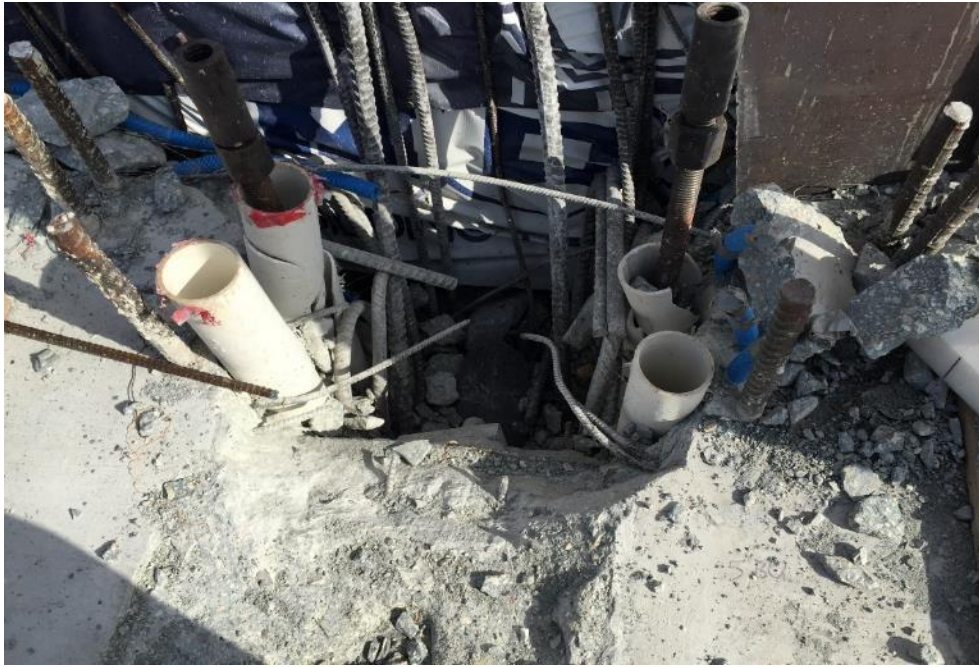
Figure 60 Concrete blow-out failure in Diaphragm II at the time of bridge collapse at the site looking north from south, March 21, 2018, by OSHA
