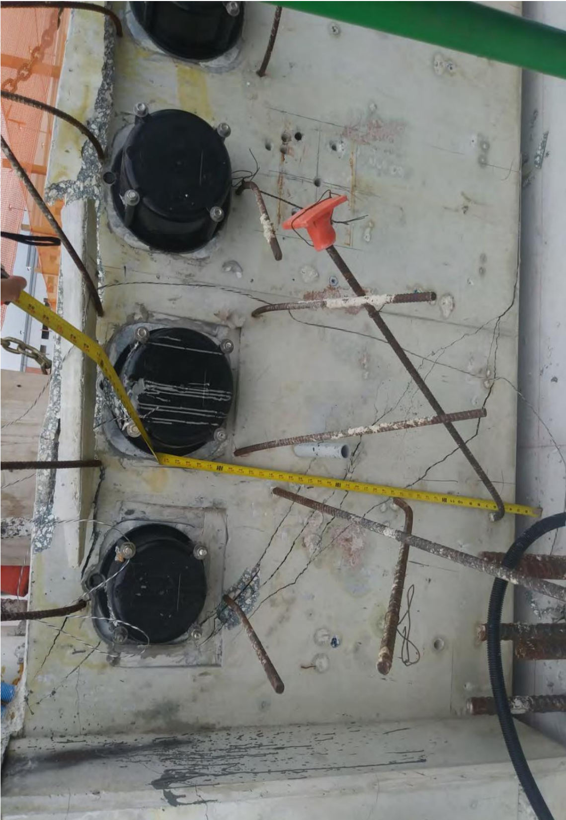
Figure 25 Cracks at the west side diaphragm II MCM email of 3/12/2018, by BPA – side face
