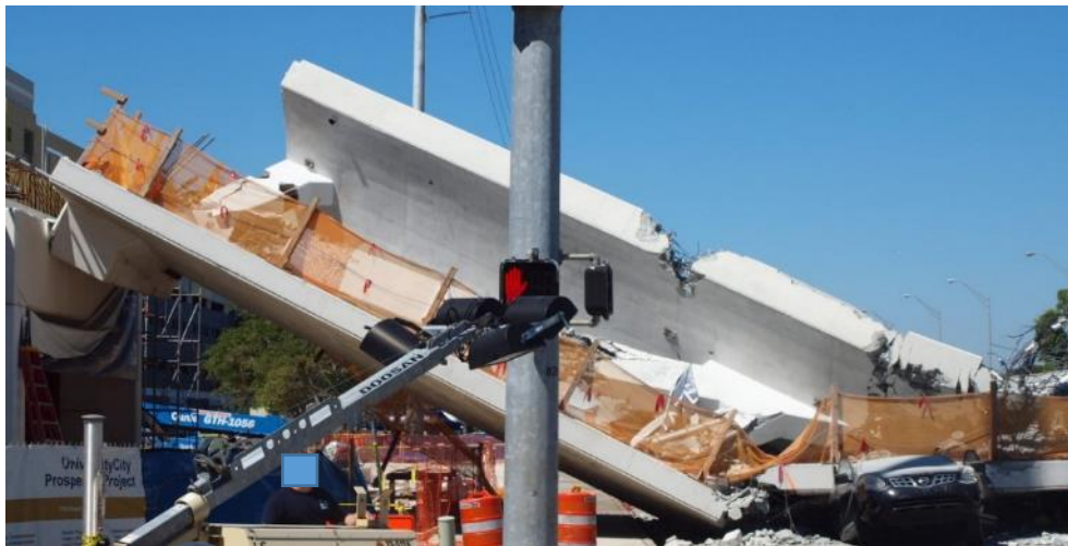
Figure 73 South end of the bridge after collapse – looking west
