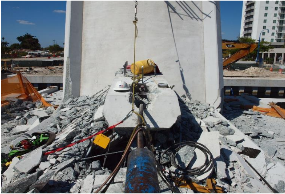
Figure 54 Northernmost blister and hydraulic jack attached to the lower PT bar of diagonal 11 after bridge collapse – front view, March 17, 2018 by OSHA
