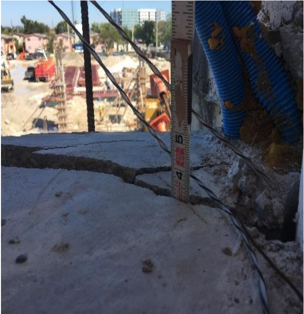
Figure 31 Notice the depth and width of cracks near column 12 at the west side of diaphragm II on 3/14/2018 by BPA
