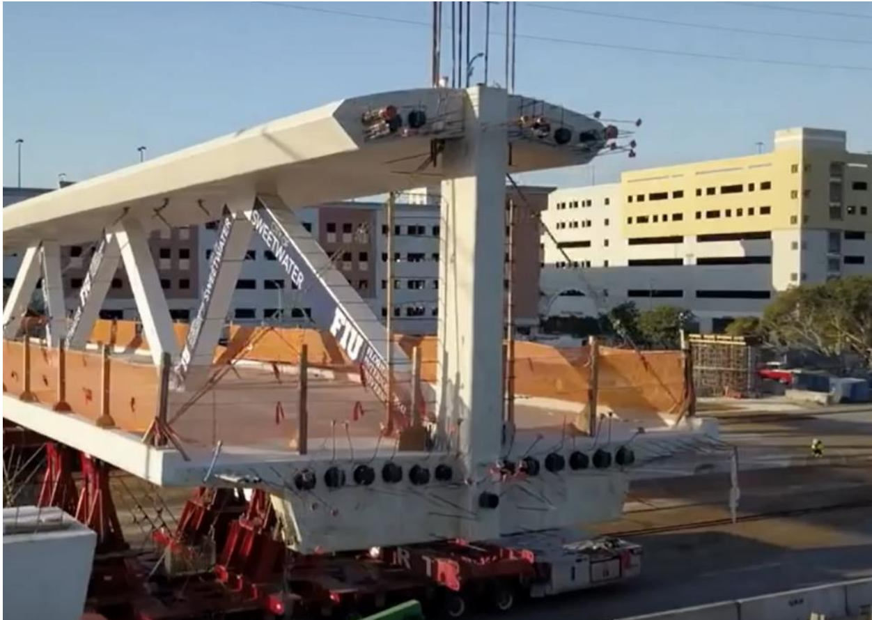
Figure 22 North end of the main span truss during transportation, generally free of cracks
