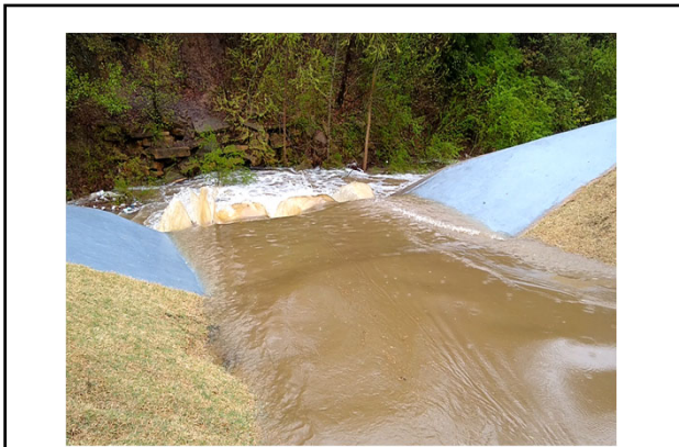
On Sunday, April 7, 2019, another significant rainfall required the Yale Road detention pond to be utilized (video).
