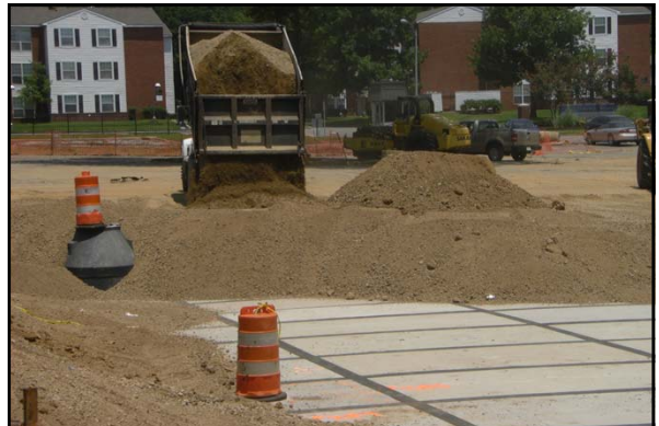
In the summer 2011, a new underground detention pond was constructed under the Central parking at the University of Memphis
