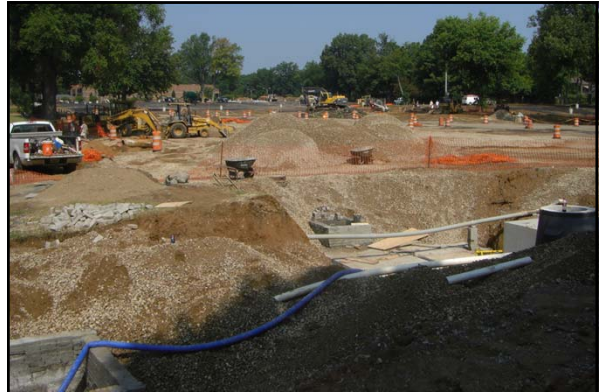
In the summer 2011, a new underground detention pond was constructed under the Central parking at the University of Memphis
