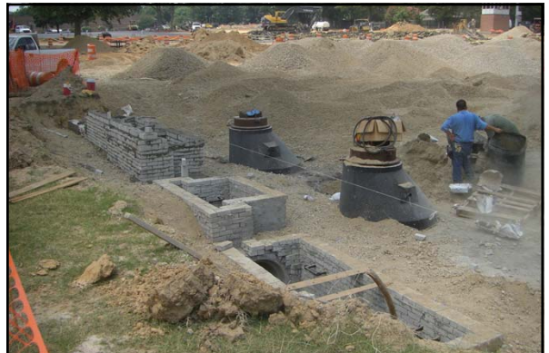
In the summer 2011, a new underground detention pond was constructed under the Central parking at the University of Memphis
