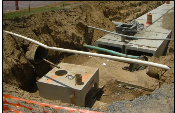
In the summer 2011, a new underground detention pond was constructed under the Central parking at the University of Memphis
