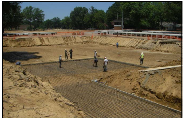
In the summer 2011, a new underground detention pond was constructed under the Central parking at the University of Memphis
