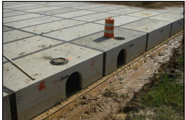
In the summer 2011, a new underground detention pond was constructed under the Central parking at the University of Memphis
