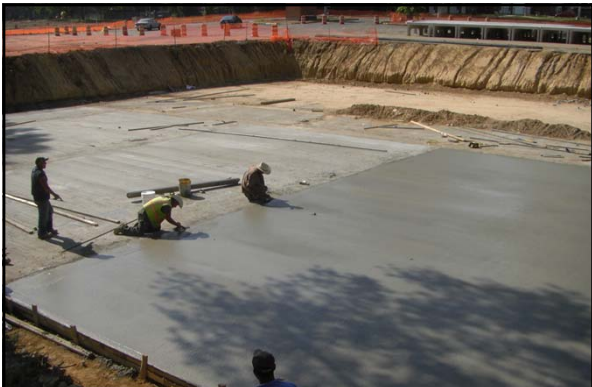
In the summer 2011, a new underground detention pond was constructed under the Central parking at the University of Memphis
