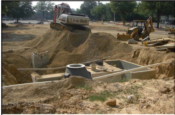
In the summer 2011, a new underground detention pond was constructed under the Central parking at the University of Memphis
