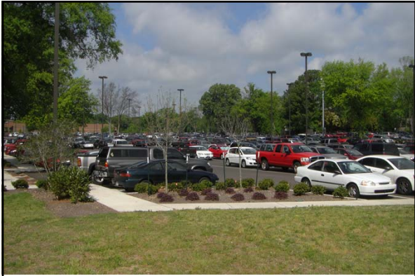
In the summer 2011, a new underground detention pond was constructed under the Central parking at the University of Memphis
