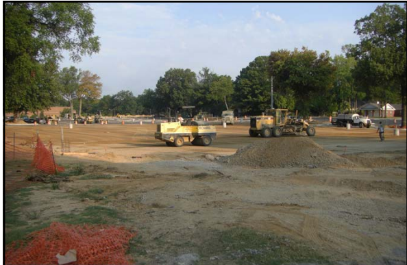
In the summer 2011, a new underground detention pond was constructed under the Central parking at the University of Memphis
