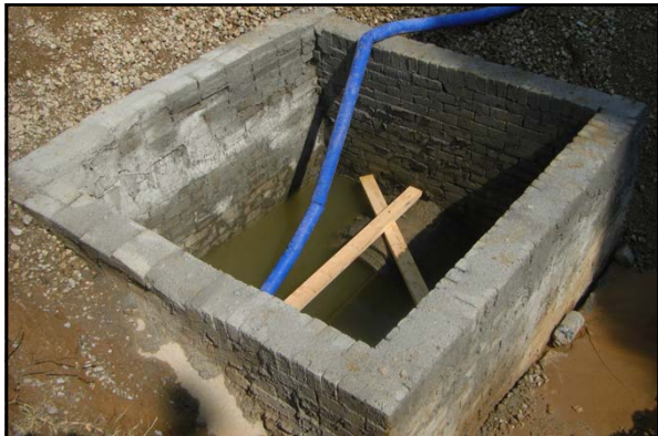
In the summer 2011, a new underground detention pond was constructed under the Central parking at the University of Memphis
