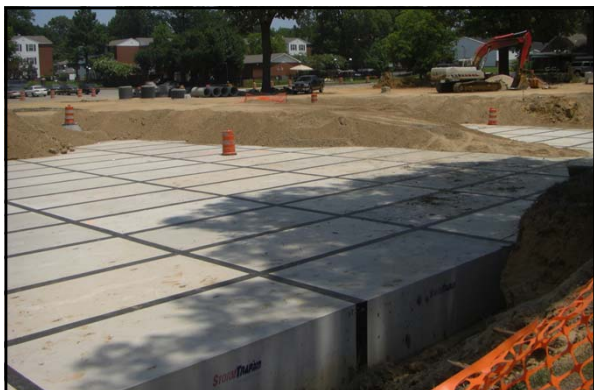
In the summer 2011, a new underground detention pond was constructed under the Central parking at the University of Memphis
