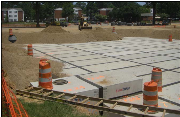
In the summer 2011, a new underground detention pond was constructed under the Central parking at the University of Memphis
