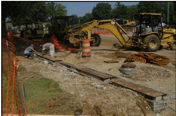
In the summer 2011, a new underground detention pond was constructed under the Central parking at the University of Memphis
