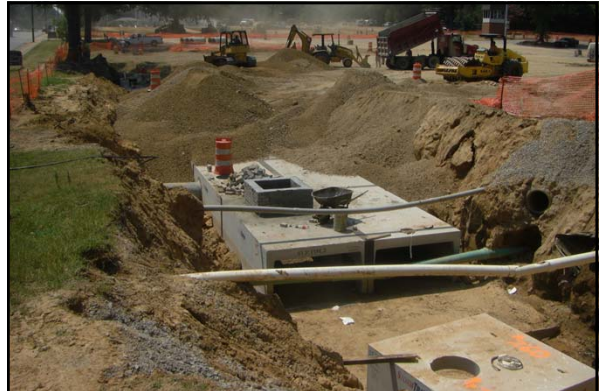
In the summer 2011, a new underground detention pond was constructed under the Central parking at the University of Memphis
