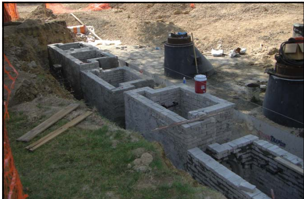
In the summer 2011, a new underground detention pond was constructed under the Central parking at the University of Memphis
