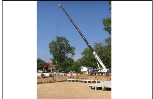
In the summer 2011, a new underground detention pond was constructed under the Central parking at the University of Memphis
