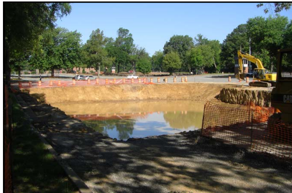
In the summer 2011, a new underground detention pond was constructed under the Central parking at the University of Memphis
