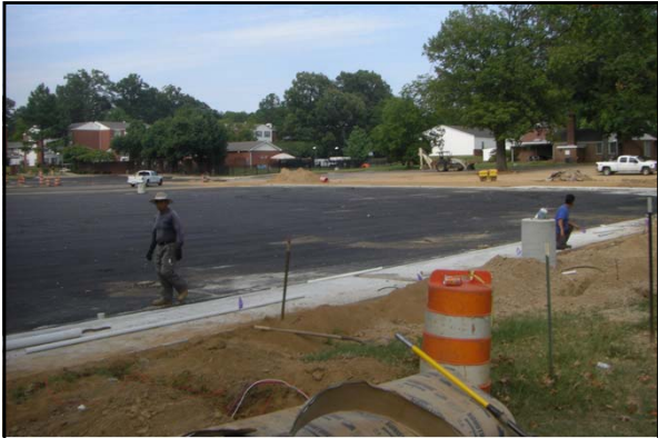
In the summer 2011, a new underground detention pond was constructed under the Central parking at the University of Memphis
