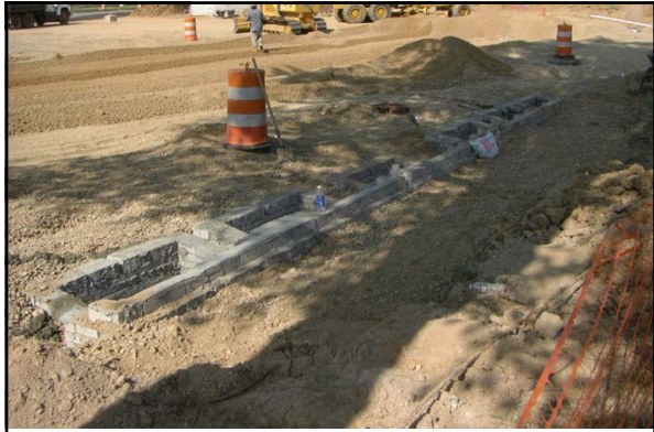
In the summer 2011, a new underground detention pond was constructed under the Central parking at the University of Memphis
