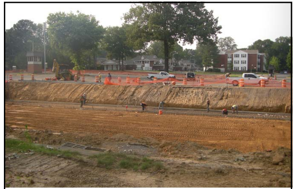
In the summer 2011, a new underground detention pond was constructed under the Central parking at the University of Memphis
