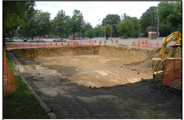
In the summer 2011, a new underground detention pond was constructed under the Central parking at the University of Memphis
