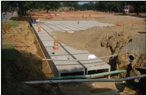
In the summer 2011, a new underground detention pond was constructed under the Central parking at the University of Memphis
