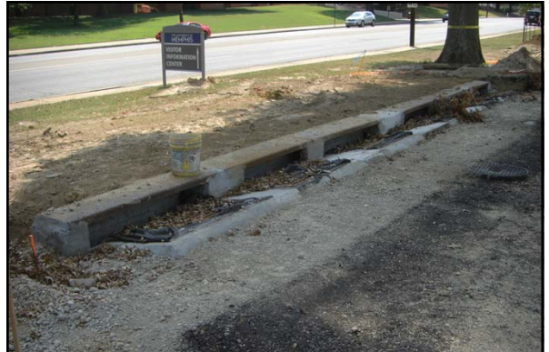
In the summer 2011, a new underground detention pond was constructed under the Central parking at the University of Memphis
