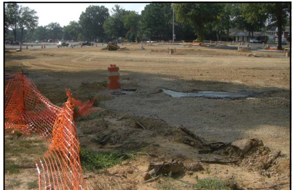
In the summer 2011, a new underground detention pond was constructed under the Central parking at the University of Memphis
