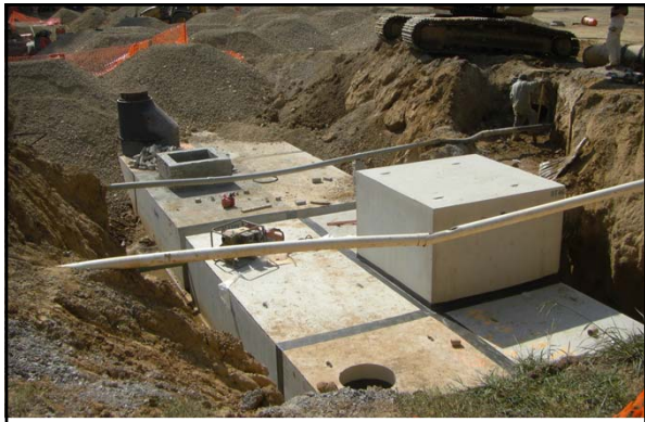
In the summer 2011, a new underground detention pond was constructed under the Central parking at the University of Memphis
