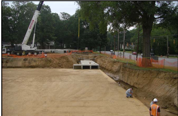
In the summer 2011, a new underground detention pond was constructed under the Central parking at the University of Memphis
