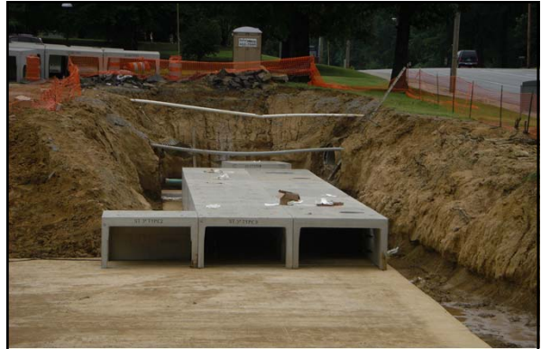
In the summer 2011, a new underground detention pond was constructed under the Central parking at the University of Memphis
