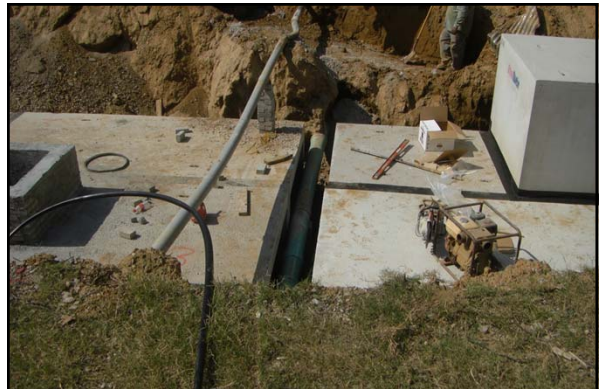
In the summer 2011, a new underground detention pond was constructed under the Central parking at the University of Memphis
