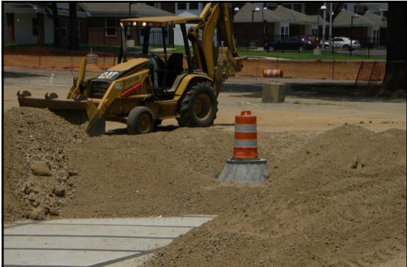
In the summer 2011, a new underground detention pond was constructed under the Central parking at the University of Memphis
