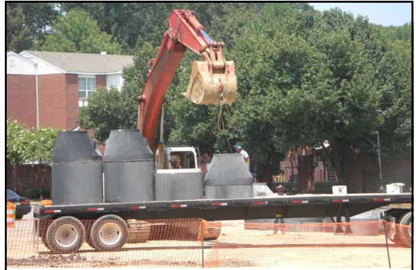
In the summer 2011, a new underground detention pond was constructed under the Central parking at the University of Memphis
