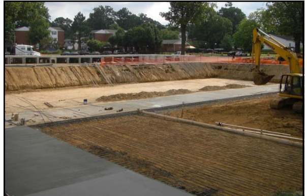
In the summer 2011, a new underground detention pond was constructed under the Central parking at the University of Memphis
