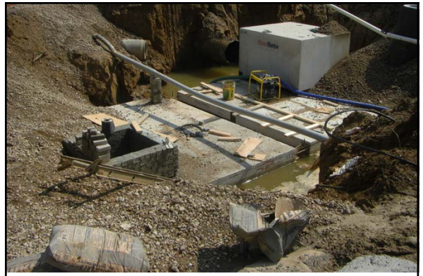
In the summer 2011, a new underground detention pond was constructed under the Central parking at the University of Memphis
