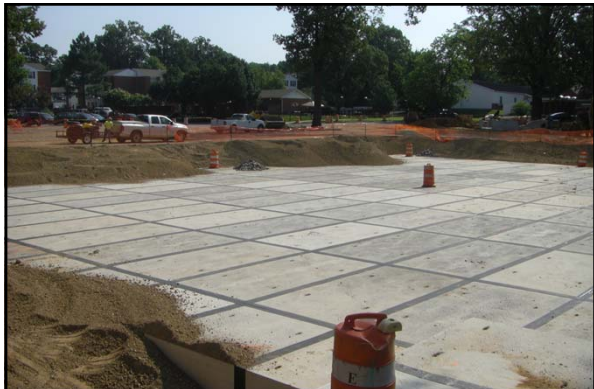
In the summer 2011, a new underground detention pond was constructed under the Central parking at the University of Memphis
