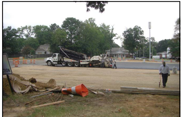
In the summer 2011, a new underground detention pond was constructed under the Central parking at the University of Memphis
