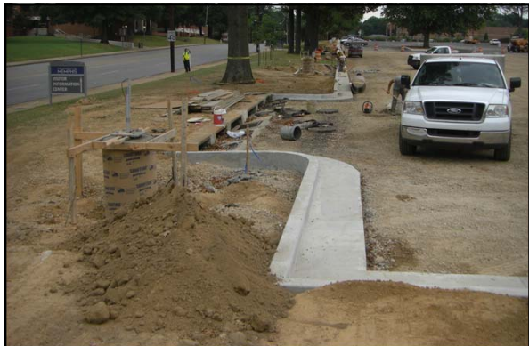
In the summer 2011, a new underground detention pond was constructed under the Central parking at the University of Memphis
