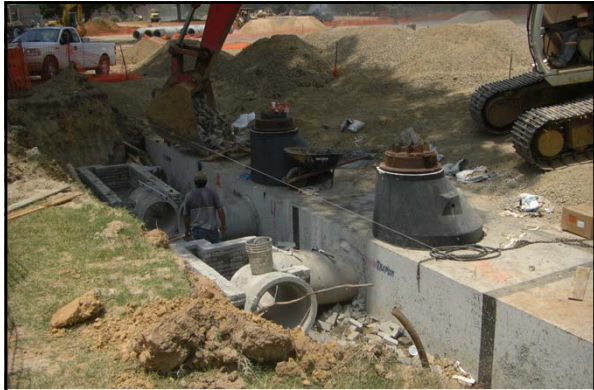
In the summer 2011, a new underground detention pond was constructed under the Central parking at the University of Memphis
