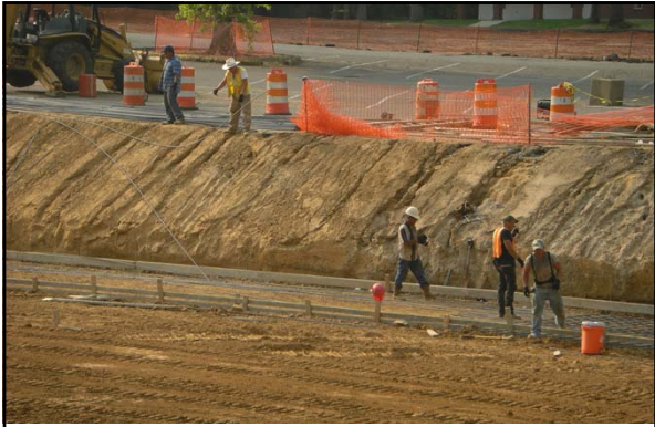
In the summer 2011, a new underground detention pond was constructed under the Central parking at the University of Memphis
