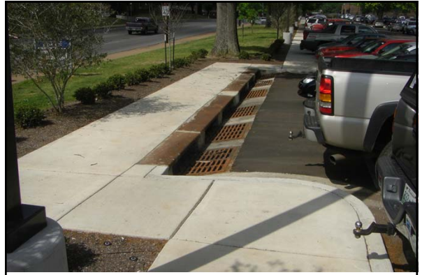
In the summer 2011, a new underground detention pond was constructed under the Central parking at the University of Memphis
