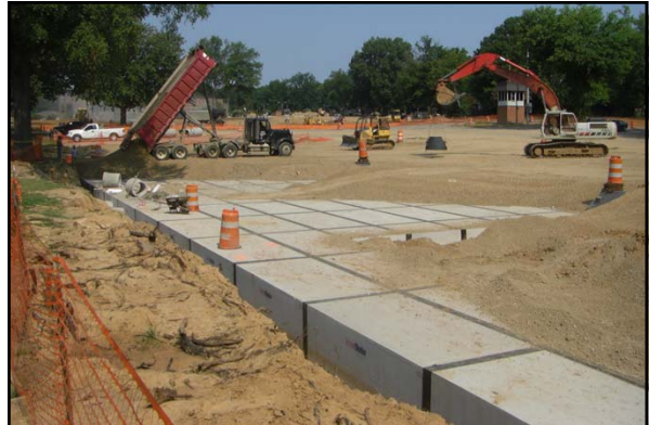
In the summer 2011, a new underground detention pond was constructed under the Central parking at the University of Memphis
