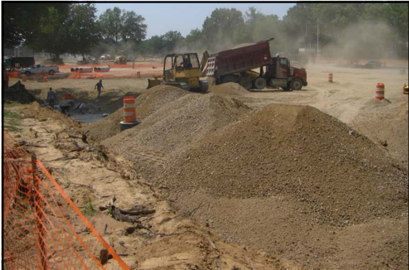
In the summer 2011, a new underground detention pond was constructed under the Central parking at the University of Memphis
