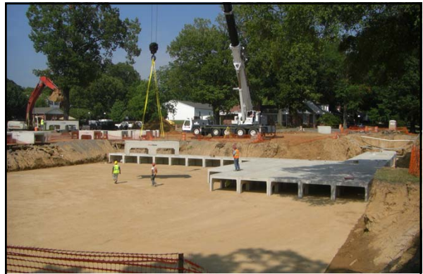
In the summer 2011, a new underground detention pond was constructed under the Central parking at the University of Memphis
