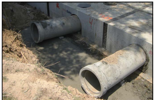
In the summer 2011, a new underground detention pond was constructed under the Central parking at the University of Memphis
