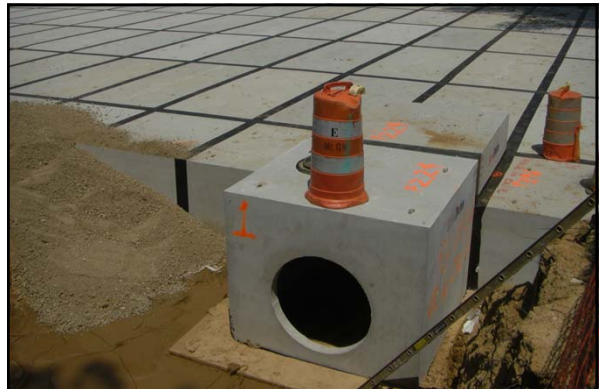
In the summer 2011, a new underground detention pond was constructed under the Central parking at the University of Memphis
