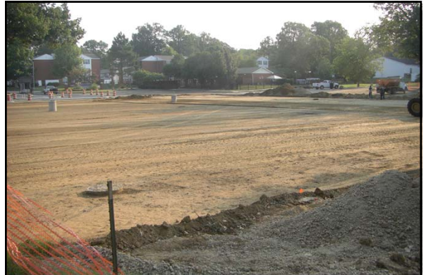
In the summer 2011, a new underground detention pond was constructed under the Central parking at the University of Memphis
