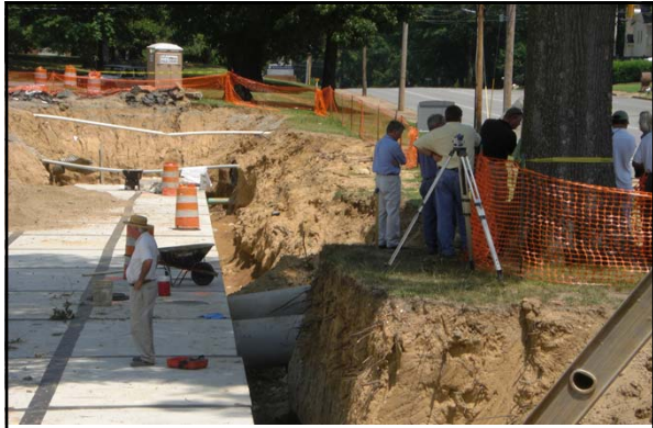
In the summer 2011, a new underground detention pond was constructed under the Central parking at the University of Memphis
