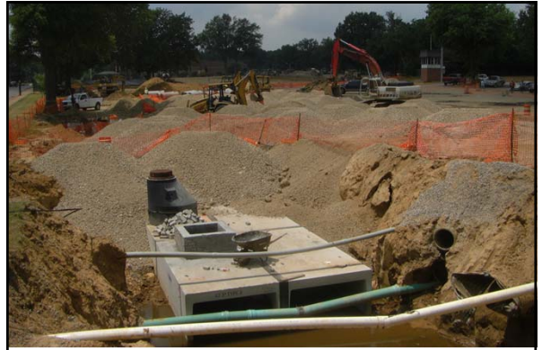
In the summer 2011, a new underground detention pond was constructed under the Central parking at the University of Memphis
