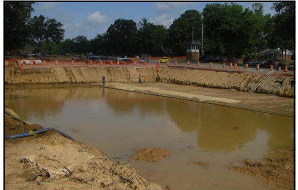
In the summer 2011, a new underground detention pond was constructed under the Central parking at the University of Memphis
