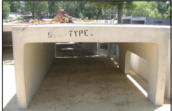
In the summer 2011, a new underground detention pond was constructed under the Central parking at the University of Memphis
