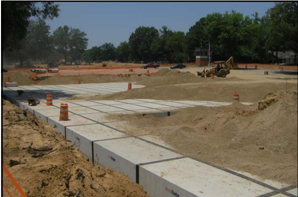
In the summer 2011, a new underground detention pond was constructed under the Central parking at the University of Memphis
