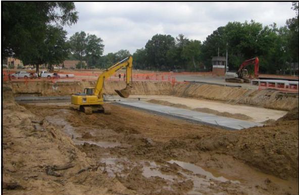
In the summer 2011, a new underground detention pond was constructed under the Central parking at the University of Memphis
