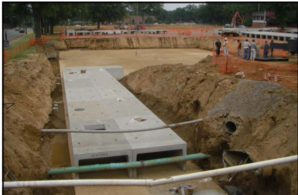
In the summer 2011, a new underground detention pond was constructed under the Central parking at the University of Memphis
