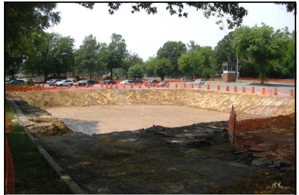
In the summer 2011, a new underground detention pond was constructed under the Central parking at the University of Memphis
