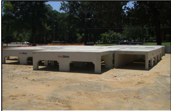
In the summer 2011, a new underground detention pond was constructed under the Central parking at the University of Memphis
