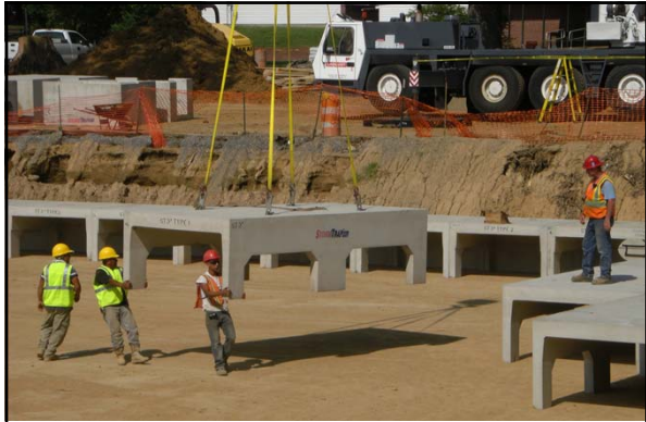
In the summer 2011, a new underground detention pond was constructed under the Central parking at the University of Memphis
