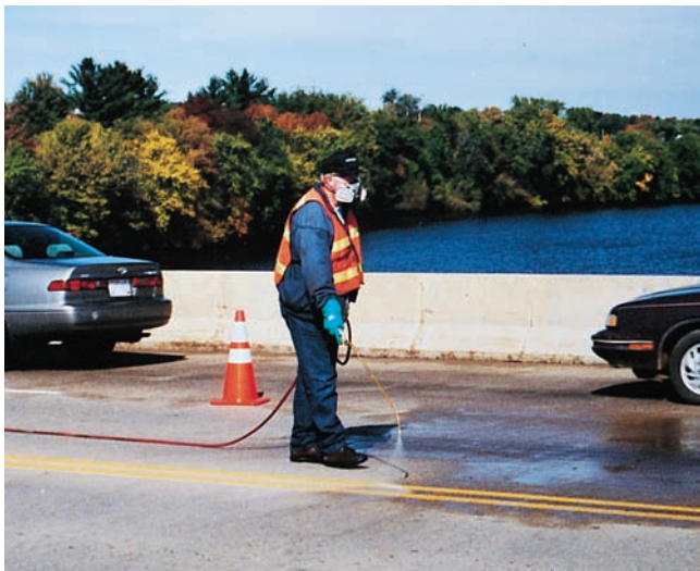
Figure 15-13. Penetrating sealers help protect reinforcing steel in bridge decks from corrosion due to chloride infiltration without reducing surface friction.
