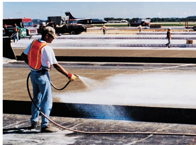
Figure 15-8. Liquid membrane-forming curing compounds should be applied with uniform and adequate coverage over the entire surface and edges for effective, extended curing of concrete.
