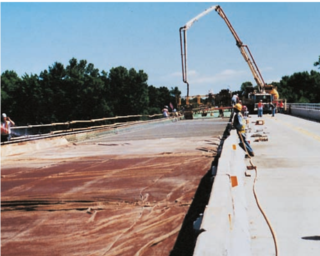
Figure 15-1. Curing should begin as soon as the concrete stiffens enough to prevent marring or erosion of the surface. Burlap sprayed with water is an effective method for moist curing.
