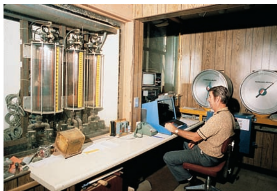
Figure 7-21. Liquid admixture dispenser at a ready mix plant provides accurate volumetric measurement of admixtures.
