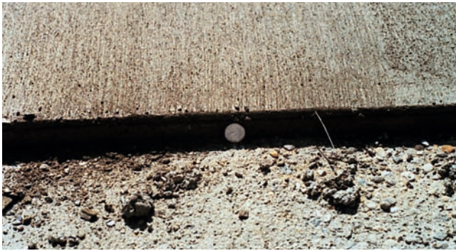
Figure 7-8. Plasticized, flowing concrete is easily placed in thin sections such as this bonded overlay that is not much thicker than 1.5 diameters of a quarter (shown).
