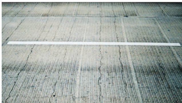
Figure 7-18. Shrinkage cracks, such as shown on this bridge deck, can be reduced with the use of good concreting practices and shrinkage reducing admixtures.
